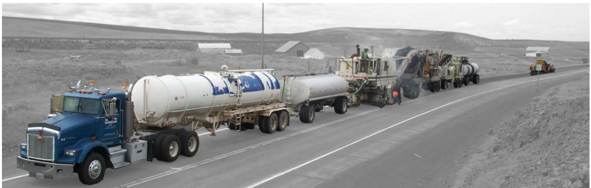
Figure MR-2.13: CIR process train (photo from the Washington State Department of Transportation).
