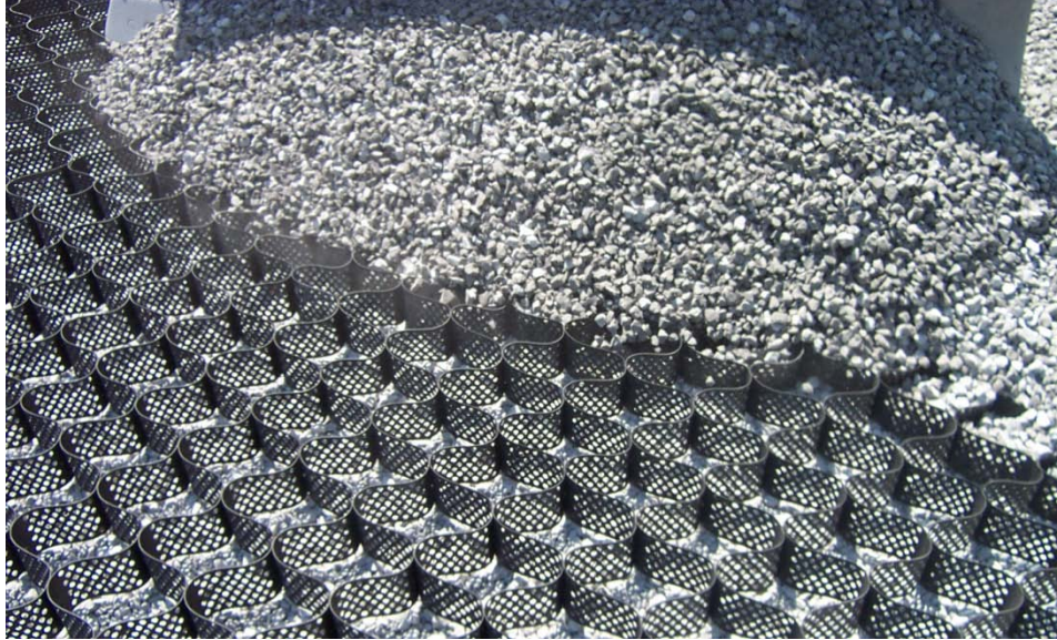
Figure PT-2.7: Table 2: Turf reinforcing grid installed in gravel parking area in Pennsylvania to alleviate ponding issues. (Blair County Conservation District, n.d.)
