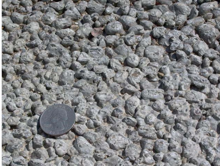
Figure PT-2.2: Porous concrete surface course in West Seattle, Washington. Quarter provided for scale. (Photo by J. Anderson)
