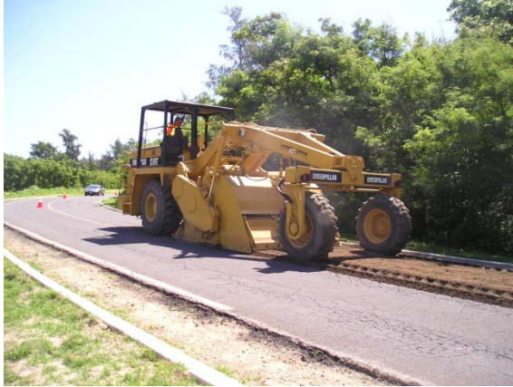
Figure MR-2.14: Road reclaimer used in FDR (photo from Grace Pacific, Inc.).
