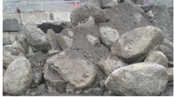
Figure PR-6.2: Boulders excavated during roadway utility work. (Bremner and City of Vancouver 2006)
