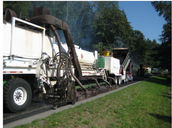
MR-2.12: HIR equipment heating and removing the top layer of existing HMA.
