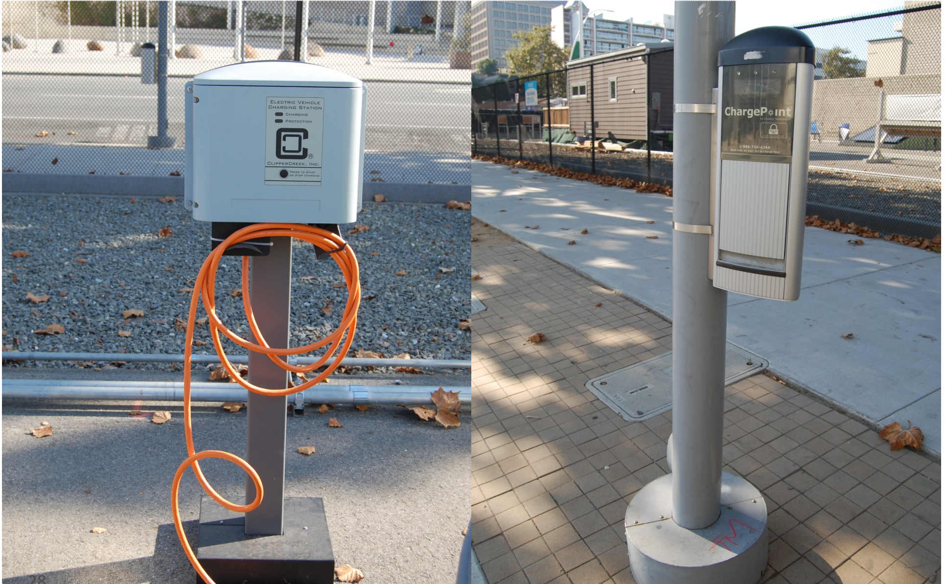
Two types of EV stations being tested by the City of San Jose, CA. Left is a demo – Right is installed.
